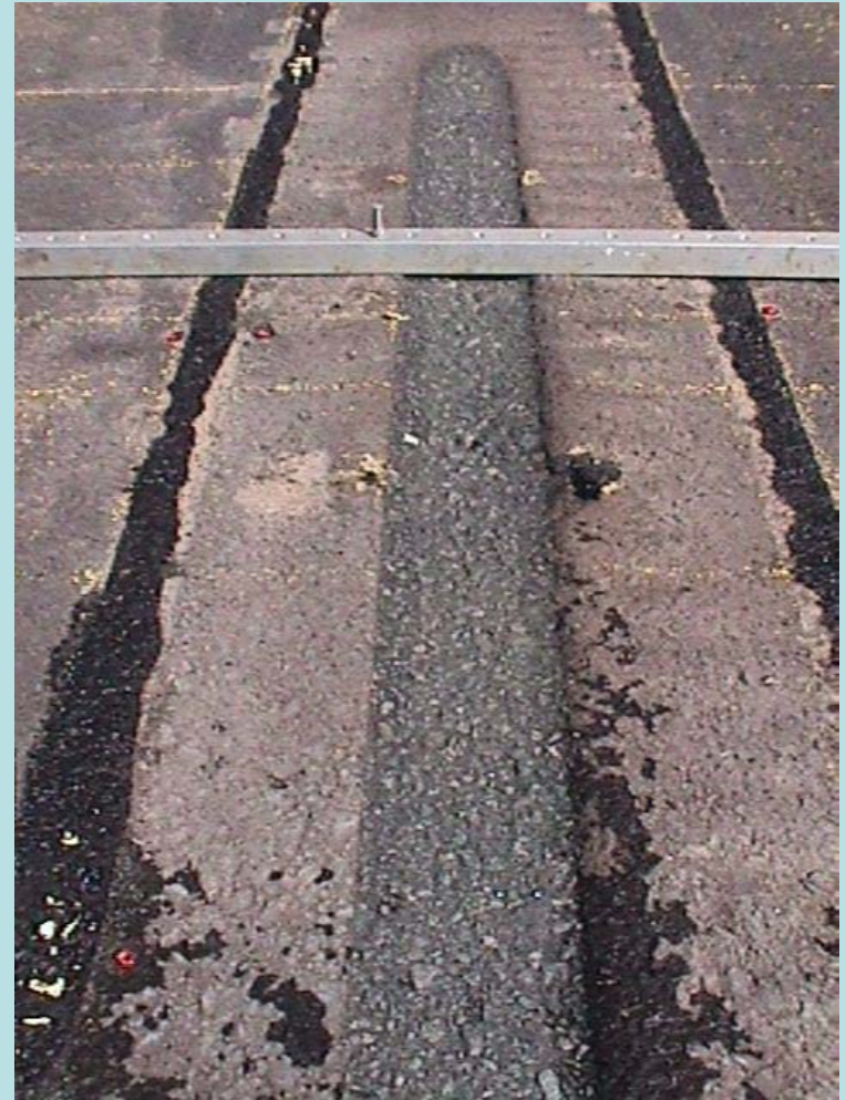
Rut after wet field testing
