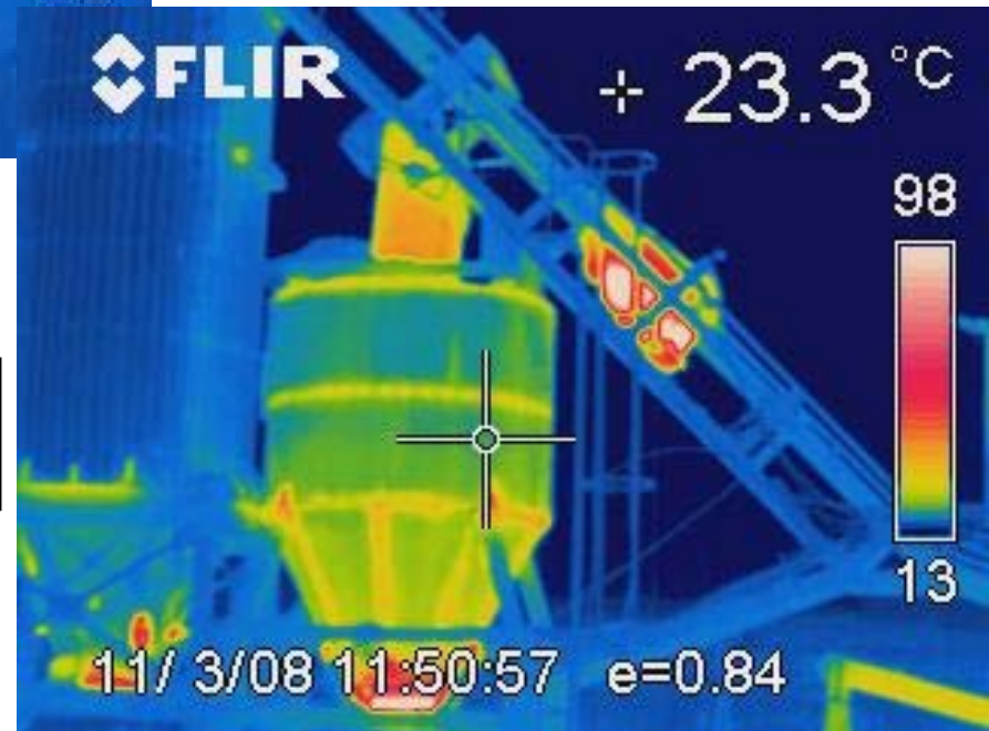
Thermal image showing the skip and hot-mix silo
