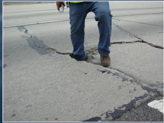
Failed Rapid Set Patches
