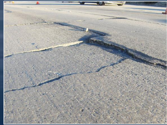
Heavily Faulted Slabs
