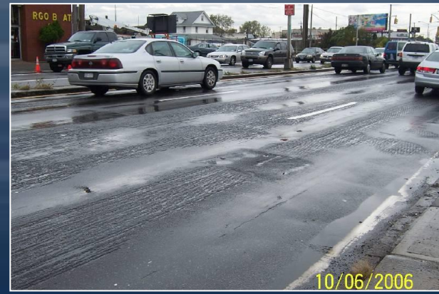
Poor Surface Drainage
