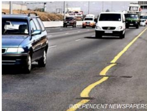
INDEPENDENT NEWSPAPERS The warping of the tarmac is clearly visible on the yellow line on the N1 near Cresta, Joburg, due to the road surface shifting. Photo: Timothy Bernard
