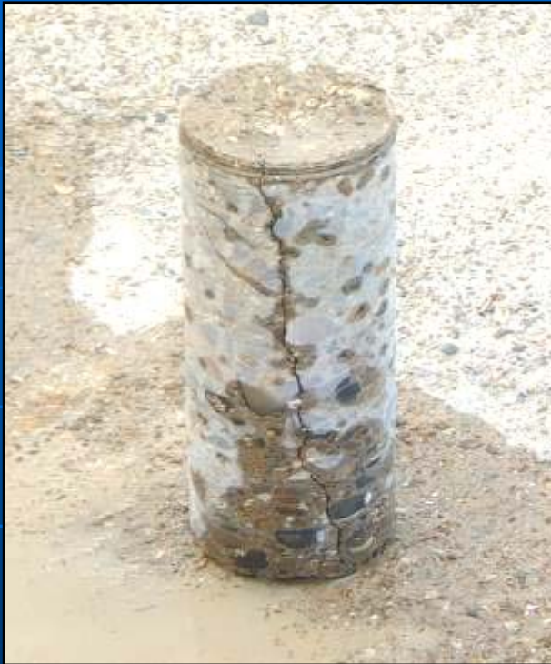
Core taken from a 450mm thick pavement
