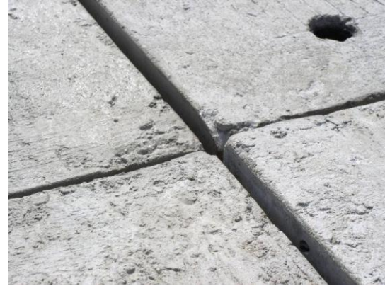
Misalignment of adjacent slabs causing surface irregularities
