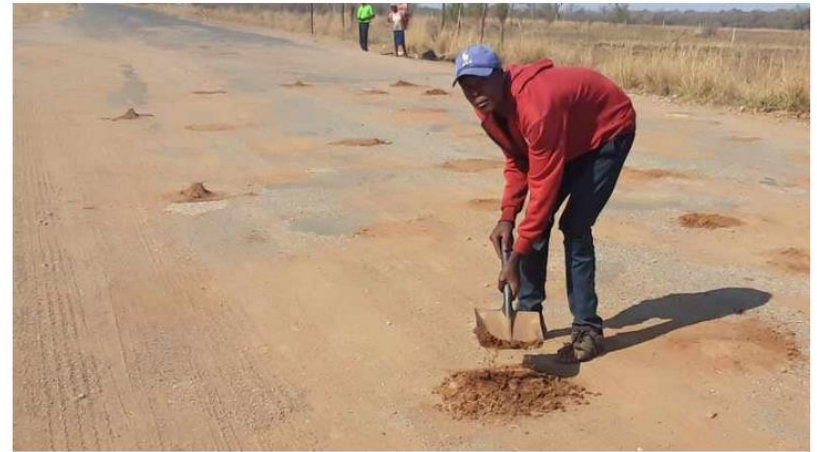
Katlego Khoza fills pothole on the D1332 with sand in Lethabong, Rustenburg in North West, the road linking Lethabong and Rustenburg has ankle-deep potholes that led to numerous horrific accidents.
